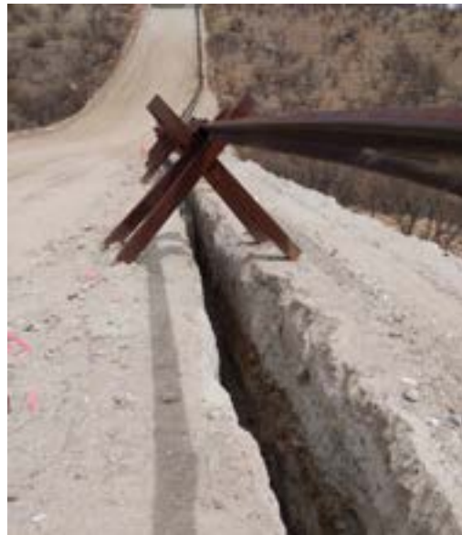
Six-foot-deep open trench created during border wall construction poses threat to natural wildlife. (Credit: Su Libby)
